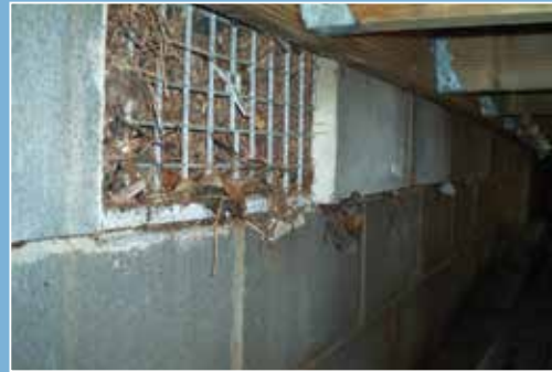
Clogged Air Vent Image credit FEMA Technical Bulletin 1, 2008
